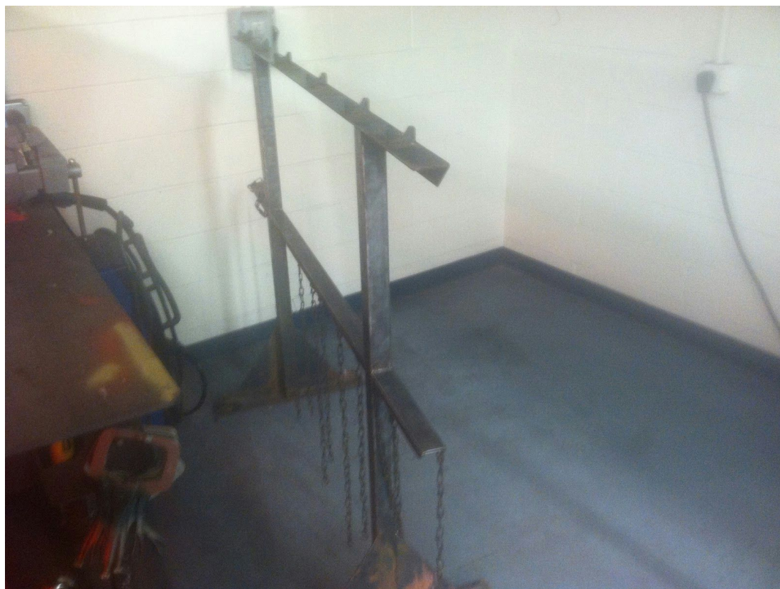
Start of the gas rack.
