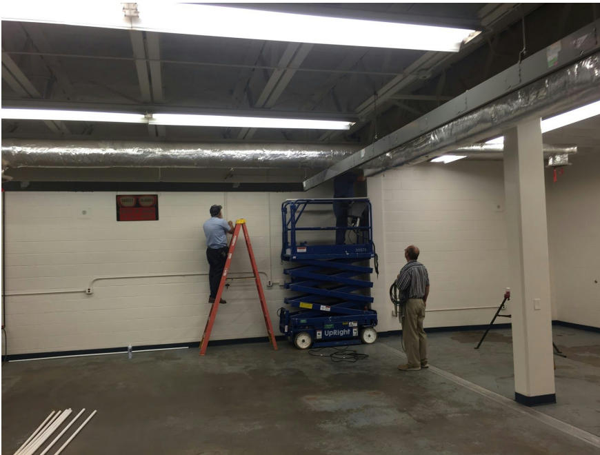
Compressed air installation
