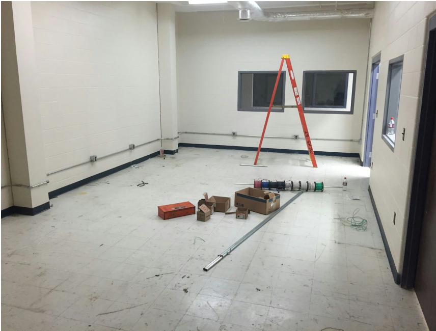
Amatrol Lab Electrical Installation
